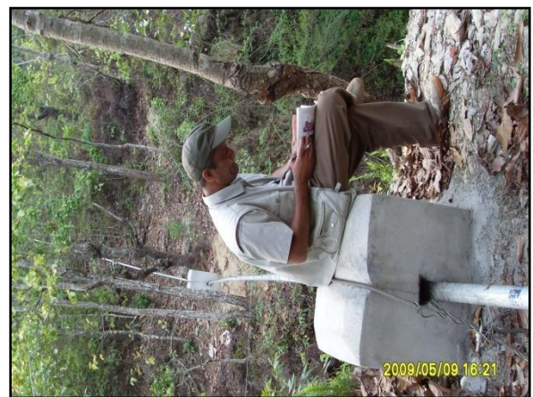
Pipe line and pass out in Masel water supply & sanitation Scheme at Masel VDC, Gorkha
