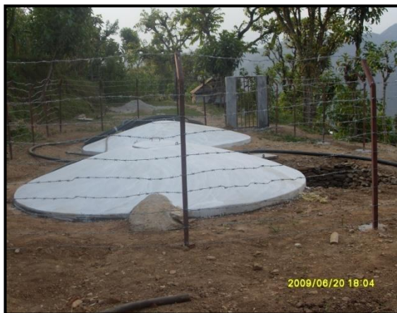
Reserve Tank at Masel water supply & sanitation Scheme at Masel VDC, Gorkha
