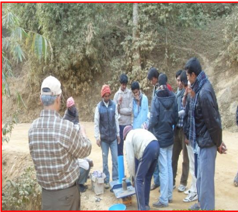
Monitoring by Mr. Lekha P. Chaulagain, CISC of Density test of road, Gorkha
